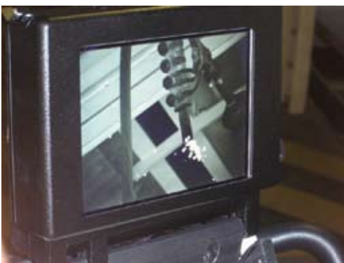
Figure 7 - A terminal end taken with a Corona Camera.
