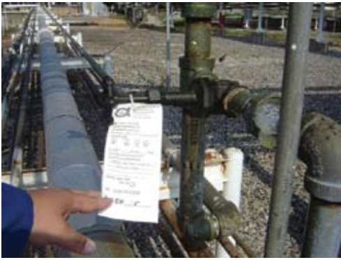
Figure 4 - Tag your leaks and photograph for referencing location and identification.
