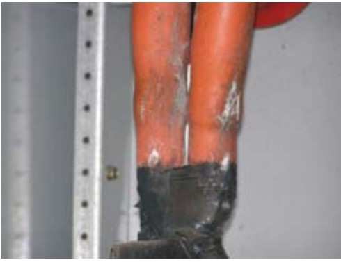
Figure 6 - White powdery residue is evidence of corona activity. This was detected using the airborne ultrasound receiver. Photo courtesy of Jim Brady, Brady Infrared Inspections, Stuart, FL.
