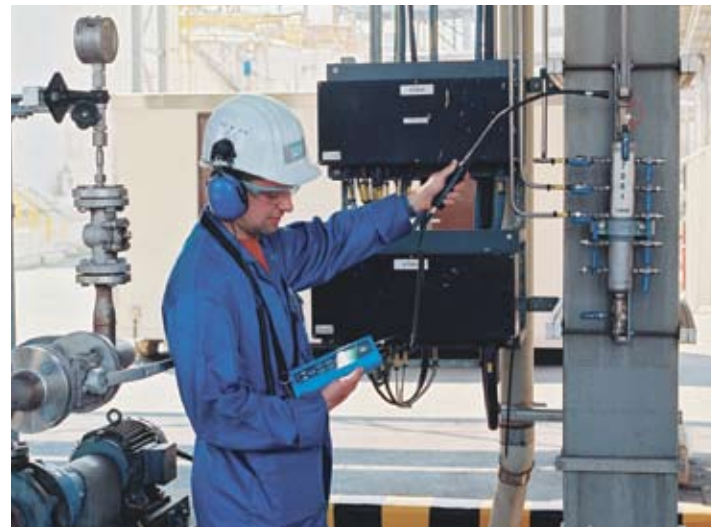
Figure 3 - Using a flexible sensor to find a compressed air leak on an instrument air line.
